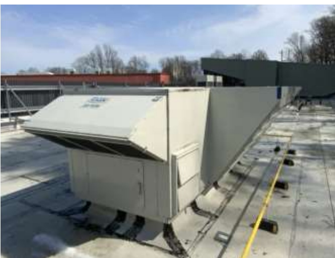
17 - PACKAGED ROOFTOP UNIT
