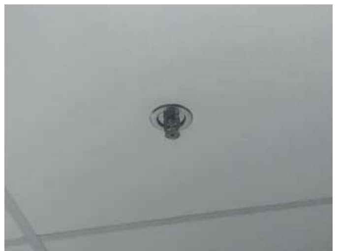
18 - FIRE SUPPRESSION SYSTEM
