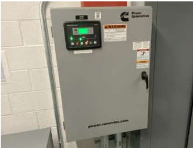
21 - AUTOMATIC TRANSFER SWITCH
