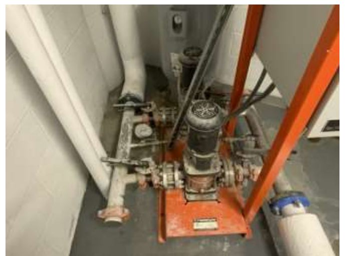
12 - BOOSTER PUMP STATION
