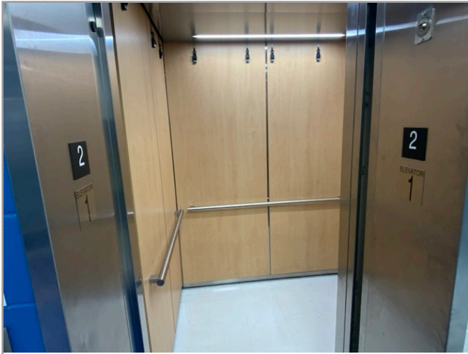
LOBBY LOOKING AT CAB
